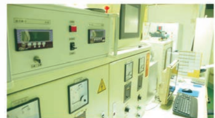
風洞實驗室 LAB OF TESTING FANS
