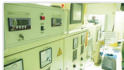
風洞實驗室 LAB OF TESTING FANS
